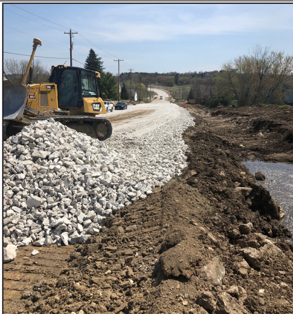
Pictured: Crews on Northview Rd in Waukesha continue to cut subgrade and undercut the roadway.
